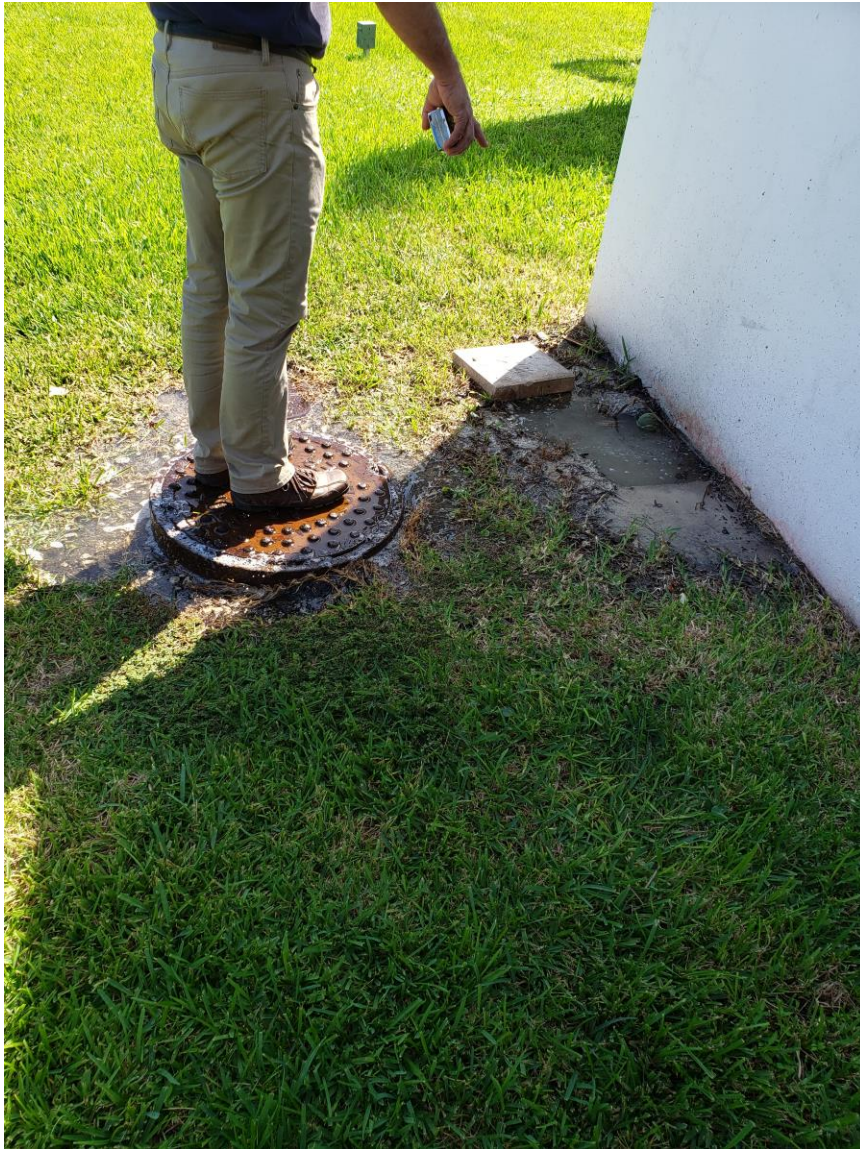
Photo 1 : (10-1-19) Manhole covers for stormwater force main at Pump Station No. 1.
