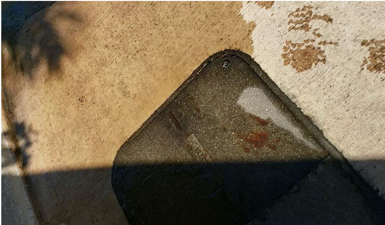
Photo 2: (10-1-19) Tidal Seepage at FPL Electric Box.
